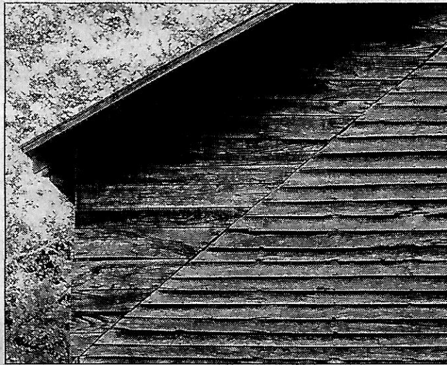
Rogers Barn closeup of roof angle addition. SPECIAL TO THE NEWS-RECORD & SENTINEL
